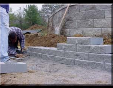
7. Additional courses of GeoStone Landscape blocks are placed upon the base course in running bond. Be consistent in setting the batter (set back) in each course.
