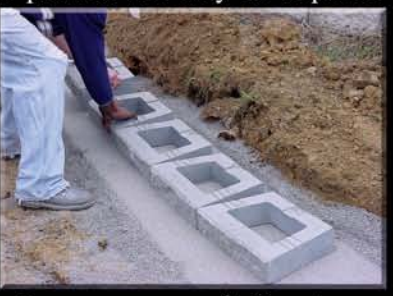
4. Base course of GeoStone Landscape blocks are placed upon compacted level rock foundation.
