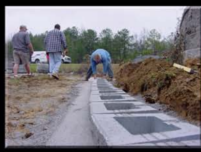
5. Blocks are aligned as desired. If wall is straight, use a string line.
