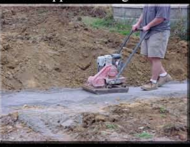
3. Foundation and leveling pad is completed with a mechanical plate tamp or hand tamp.
