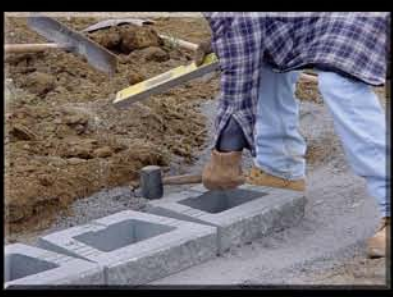
6. Finish leveling. Using a 2 foot carpenter's level and a rubber mallet, level each block front to back and side to side level with the adjoining block.
